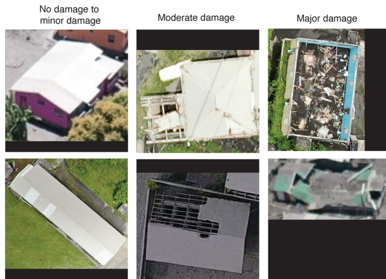
Figure 2. Example of the three damage states used in this work: No damage to minor damage, Moderate damage and, Major damage.
