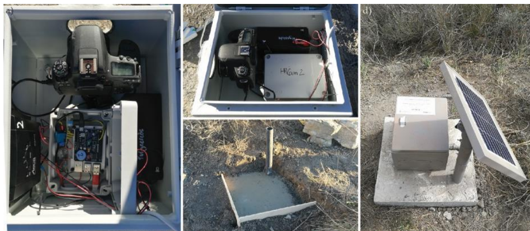
Figure 1. Images of the photogrammetric systems installed in the Puigercós site: a and b) Images showing the inside of the photogrammetric unit with part of the connections shown in Figure 3; c) Construction of the concrete base and installation of the PVC pipe for the installation of the photographic units and d) external view of the installed system.
