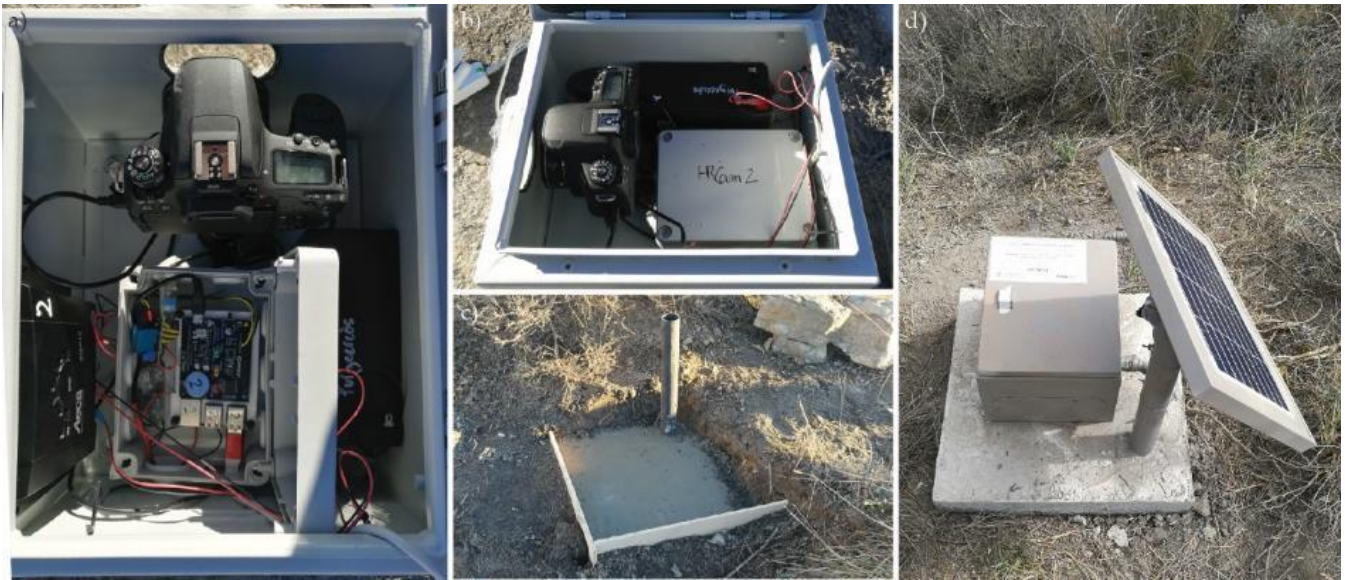
Figure 1. Images of the photogrammetric systems installed in the Puigcercós site: a and b) Images showing the inside of the photogrammetric unit with part of the connections shown in Figure 3; c) Construction of the concrete base and installation of the PVC pipe for the installation of the photographic units and d) external view of the installed system.
