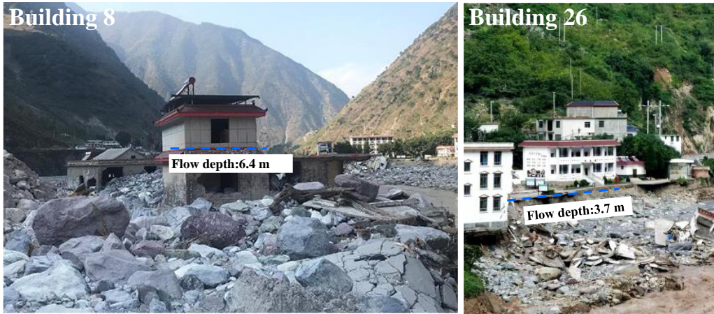
Figure 9 Simulated maximum flow depth of the dam-burst flood at the location of Buildings 8 and Building 26
