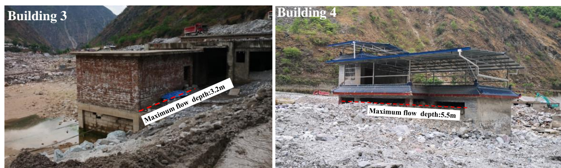
Figure 7 Simulated maximum flow depth of debris flow at the location of Building 3 and Building 4
