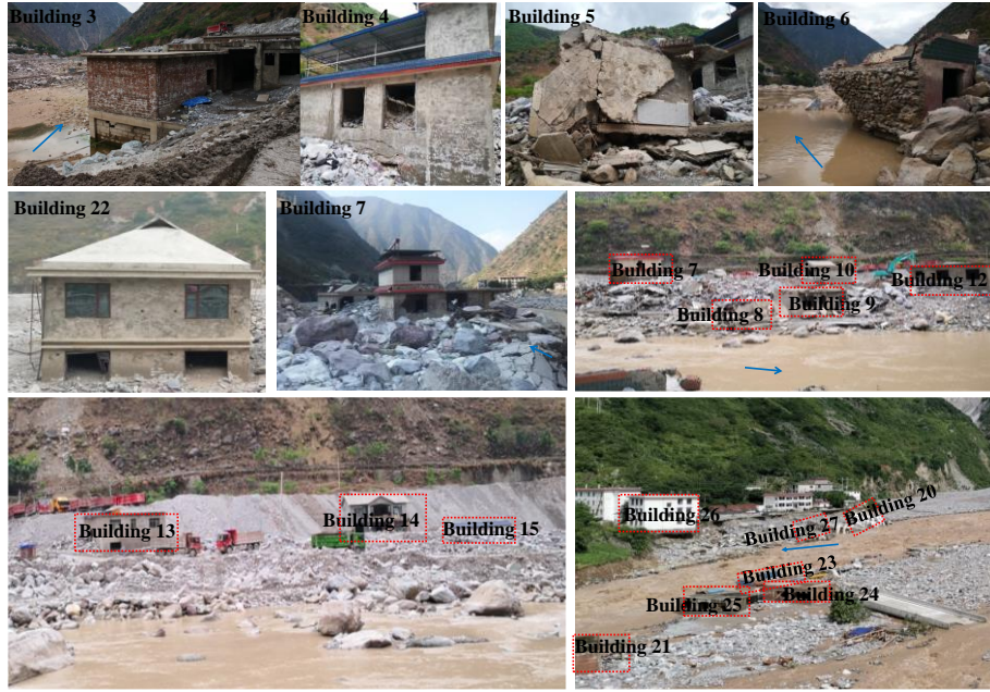
Figure 11-13 Buildings with different degrees of damage within three hazard zones.
