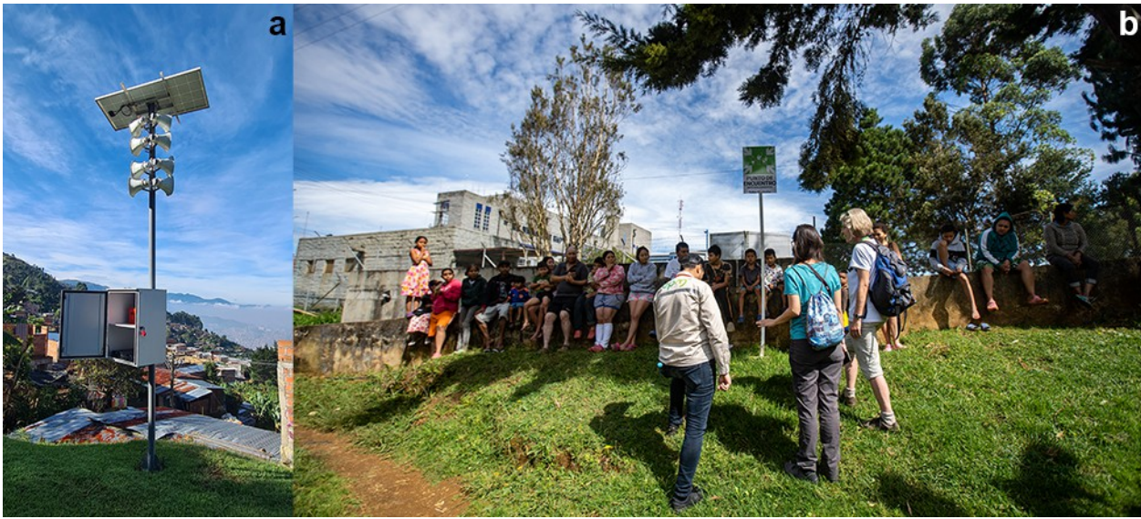
Figure 13. (a) siren system that can be manually operated and (b) residents congregate at one of the meeting points after an emergency drill.
