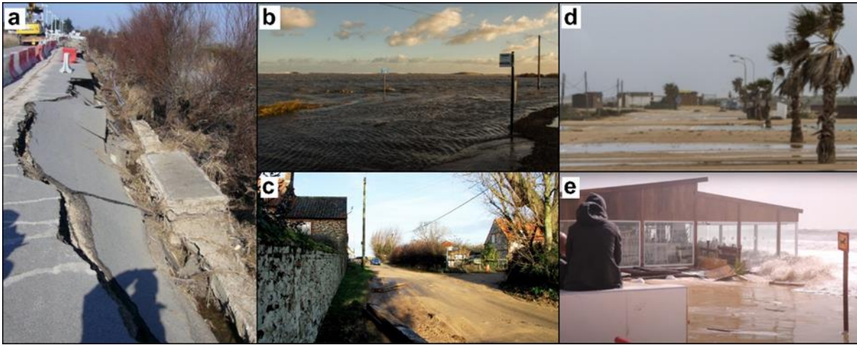
465 Figure 9: Examples of damage to roads: (a) Route de la Tranche-sur-Mer in the area of La Faute-sur-Mer (France) after the Xynthia event in February 2010; (b) Coast Rd (Salthouse, Holt) and (c) Beach Rd (Holme-next-the-Sea, Hunstanton) in the Norfolk (UK) area after the Xaver event in December 2013; (d) Carretera Playa de Camposoto in the south of the city of Cadiz (Spain) after the Emma event in March 2018. The images were retrieved from the sources of information collected in the ECFAS database of extreme events and test cases (Souto Cecon et al., 2021).
