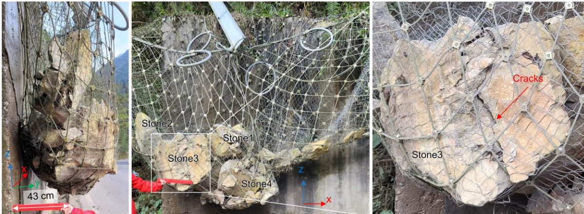
115 Figure 4: Rockfalls piled up in the net.
