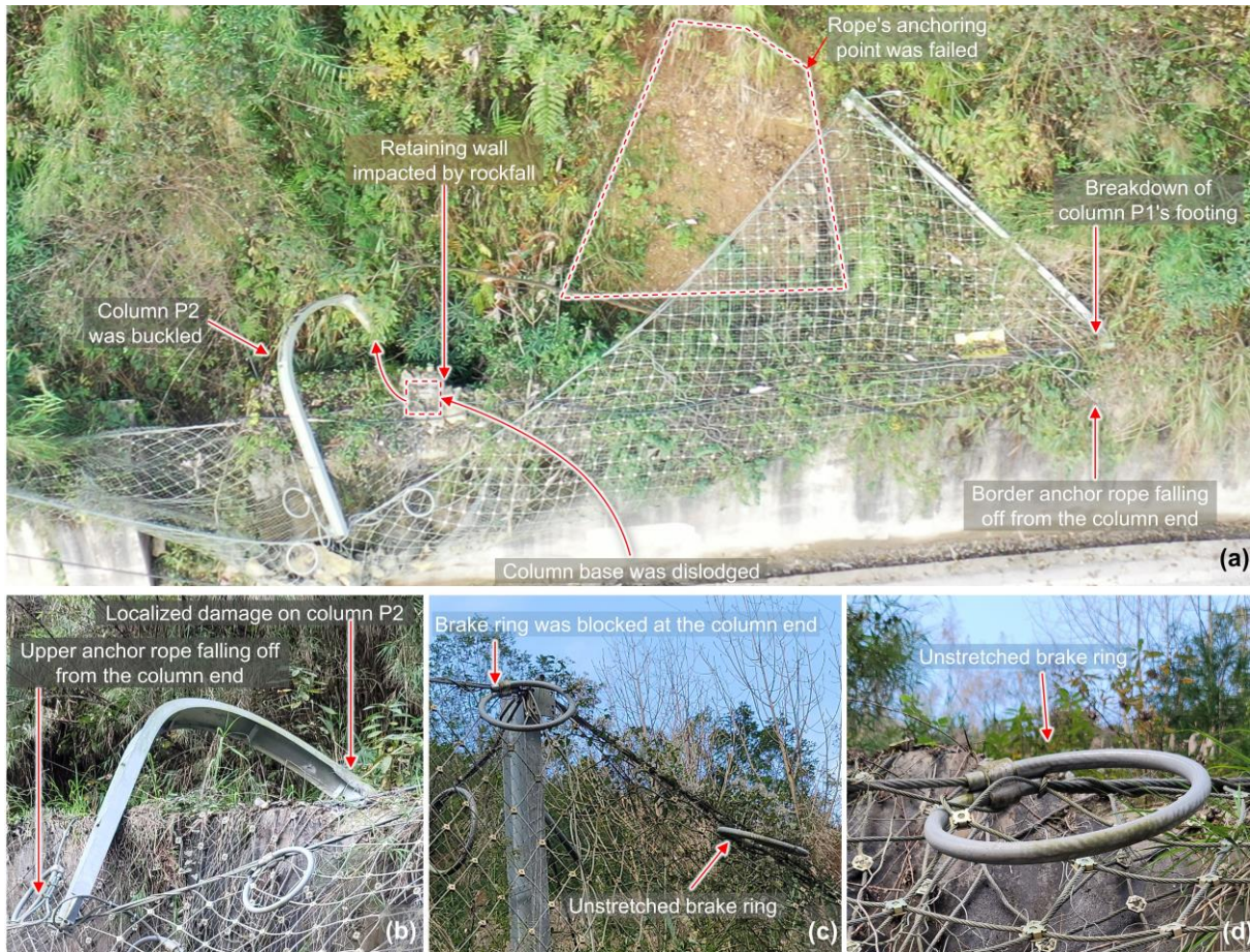
Figure 6: Damage phenomena of the flexible barrier. (a) The damaged two-span structure; (b) Failure of column P2; (c) Non-working brake rings on both sides of the column P3 end; (d) Connection relationship between the brake ring and the support rope and the steel wire rope net.
