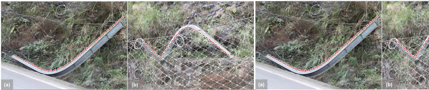
Figure 2: Steel column buckling forms of the other two flexible rockfall barrier projects: (a) "C"-shaped compression buckling and (b) "S"-shaped bending and torsion buckling.
