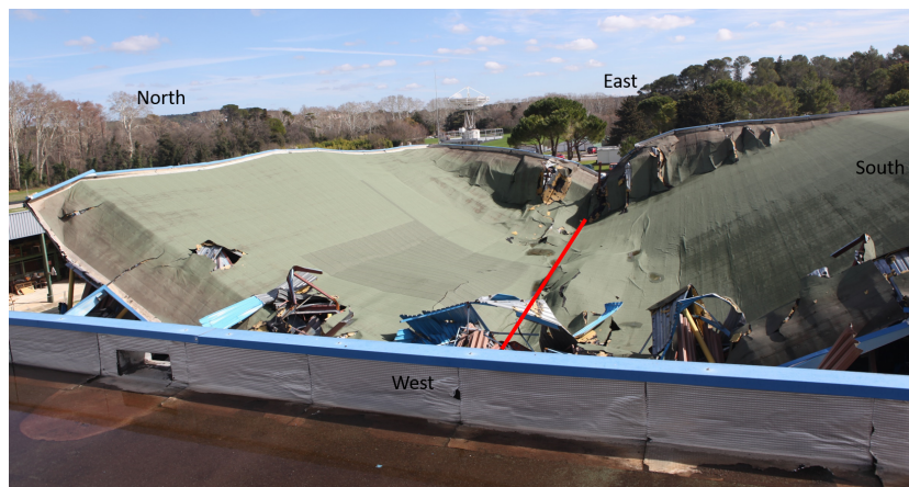
Figure 10. Overview of the damaged Irstea Cévennes building.
