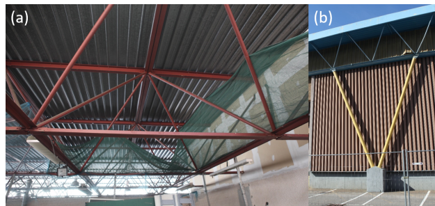
Figure 7. View of the supporting structure of the Irstea Cévennes building before its damage: (a) red-colored roof metal frame and (b) supporting tubular pylons (in yellow) along the facades.
