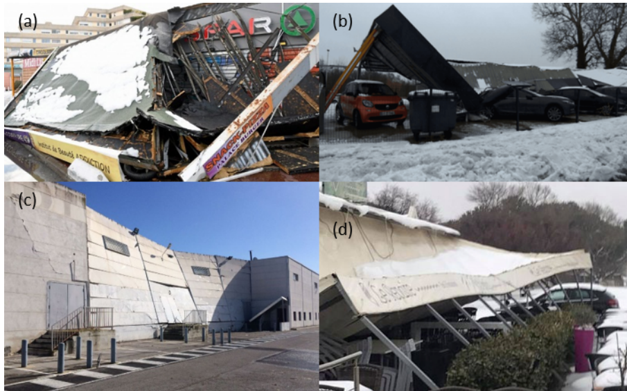
Figure 1. Roof collapses due to heavy snowfalls occurred on 28 February and 1st March 2018 in the surroundings of Montpellier, France: collapses of (a) the shopping center Estanove in Montpellier (Photo credit: ©Jean-Michel Mart), (b) a car wash station in Lattes (Photo credit: ©Le Petit Journal de Lattes), (c) the Darty store in Peyrols (Photo credit: ©France 3 LR / S. Banus) and (d) a restaurant in La Grande Motte (Photo credit: ©France 3).
