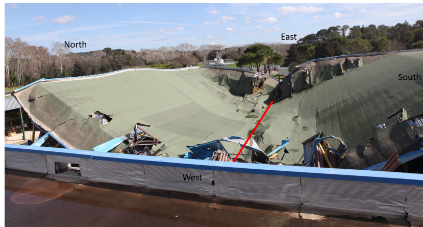
Figure 10. Overview of the damaged Irstea Cévennes building.
