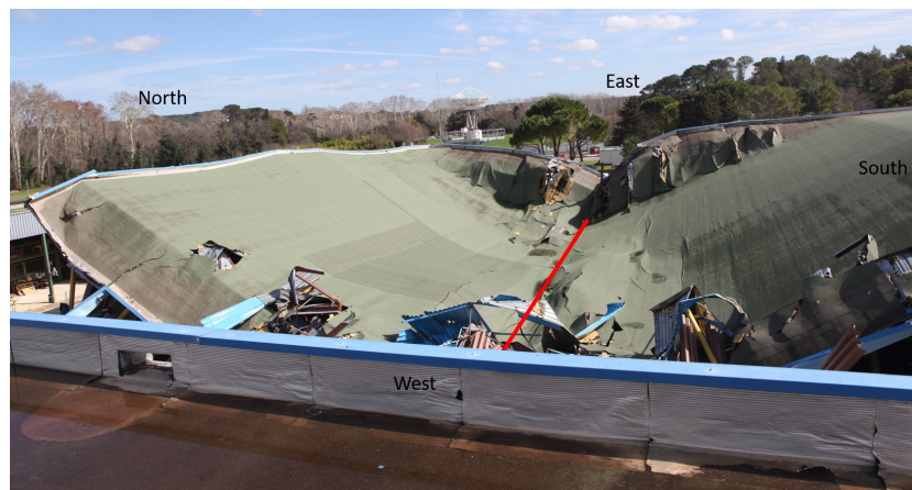
Figure 10. Overview of the damaged Irstea Cévennes building.
