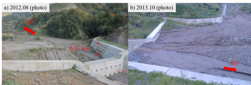
Fig. 10. The photos of dam 1 reservoir (the red single arrows showing the azimuth angle and the double arrows showing the height of the dam body)
