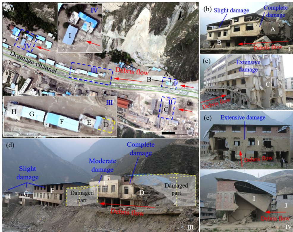
Figure 8. Distribution of damaged-buildings in Qipan gully debris flow event. Orthophoto map is from the Basic Geographic Information Center of Sichuan Province, China, 21 July 2013.
