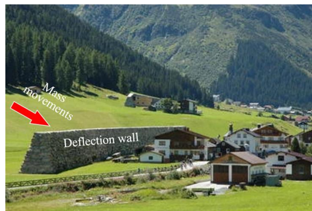
350 Figure 9. A deflection wall used to protect an entire building ensemble from the impact of medium magnitude events (Galtur Tschafein, Austria) (Holub et al., 2012).
