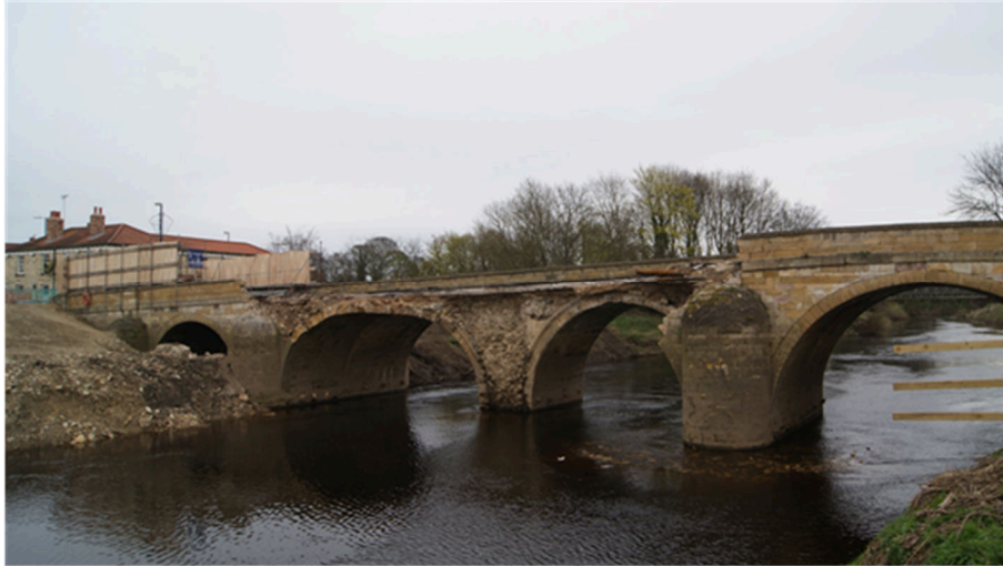
330 Figure 3. Tadcaster bridge, damaged by Storm Eva in 2015, repaired and reopened to traffic 13 months after. Bridge closure resulted in 9-mile detour of 20 minutes to reach the other side. Source: https://commons.wikimedia.org/wiki/File:Tadcaster_Bridge_closed_following_last_years_damage_(10th_April_2016)_005.JPG
