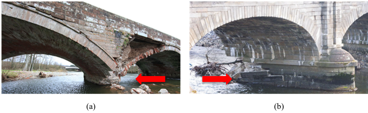
225 Figure 2. Damage of Brougham Old Bridge (a) and of Calva bridge (b), typical of many masonry arch bridges subjected to scour (Source: Cumbria Council County for (a) and Bill Harvey for (b)). Flow direction indicated by arrow.
