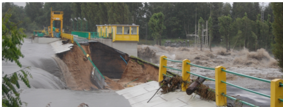
Figure 7. View from the right bank. Behind the concrete structure, an immense outflow is visible after the abutment had collapsed. Water level in the reservoir ca. 210.60 m a.s.l.
