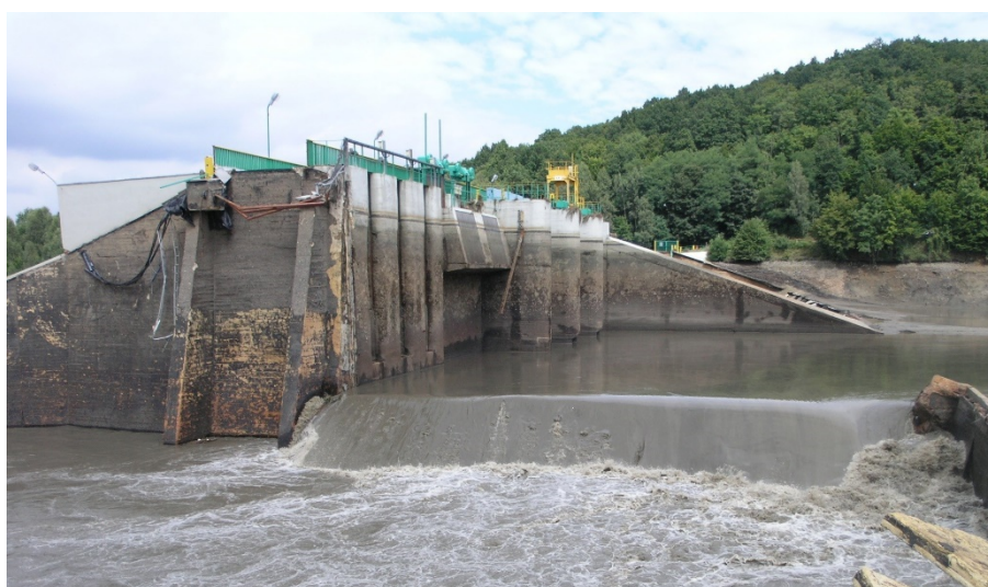
Figure 8. Broken left retaining wall of the control structure
