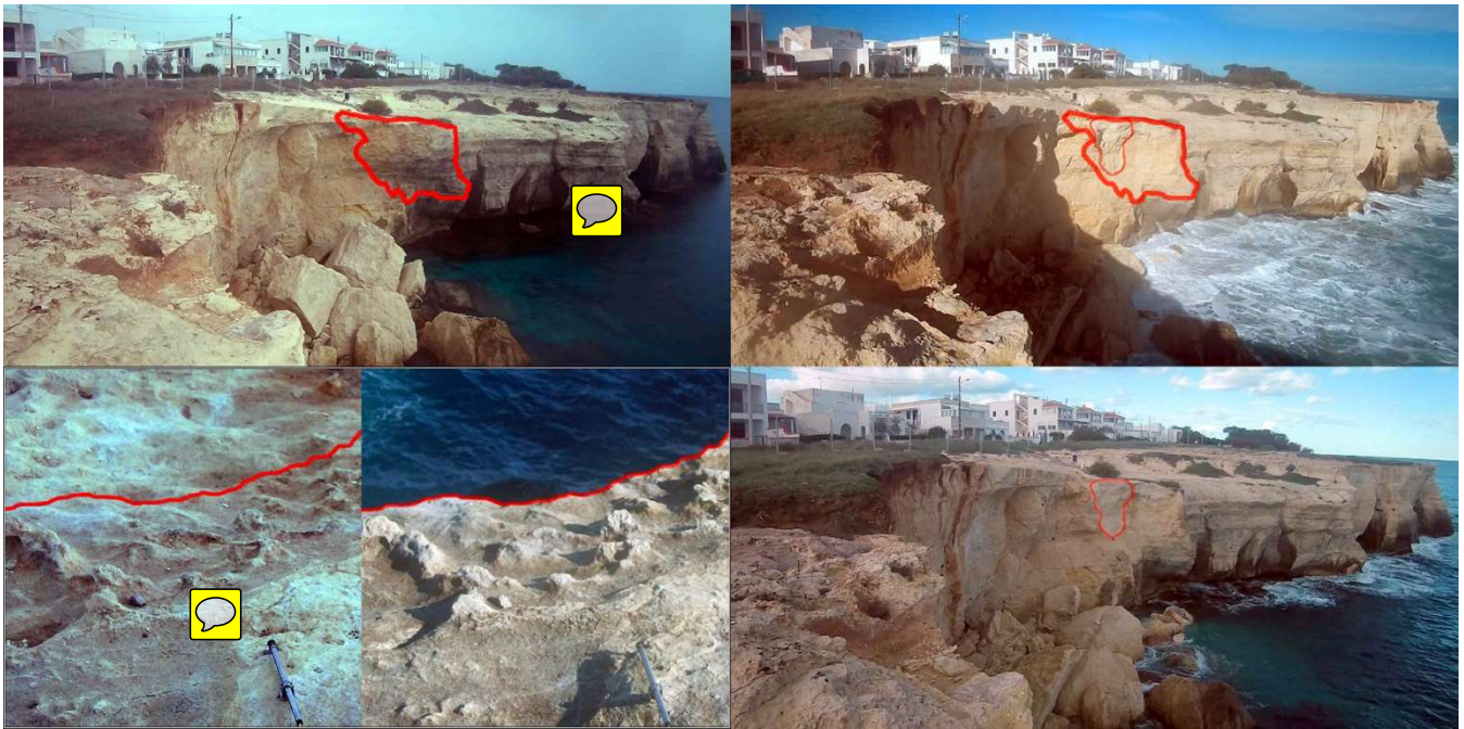
170 Figure 3: the second rockfall (marked with “B” on figure 2) – Top left image shows the cliff as it was on 4 December 2020 and the top right image shows as it was on the morning of the 7 December 2020, after the main collapse (marked by the thick red line). Bottom right images shows the cliff as it was on the 8 December 2020, after a minor rockfall (marked by the thin red line). On the bottom left part, two smaller images that shows the collapse from another point of view (the main camera) both before the rockfall (on the left) and after it (on the right). On those images, the newly installed automatic crack-meter is also visible.
