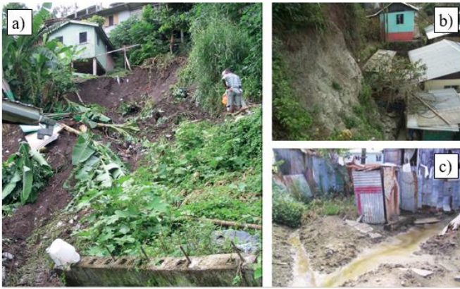
330 Figure 1: Examples of informal housing affecting land stability. The image (a) and (b) show examples of unsupported cut slopes, respectively in Saint Lucia (Caribbean) and Dumsi Pakha (Kalimpong, India). The image (c) shows the effect of lack of water management in an informal community of Saint Lucia (Caribbean). From the blog AGU landslides: https://blogs.agu.org/landslideblog/2016/03/14/managing-urban-landslides-1/ From the blog Save the Hills ( http://savethehills.blogspot.com/ ) and the community based project Mosaic (Anderson and Holcombe, 2013)
