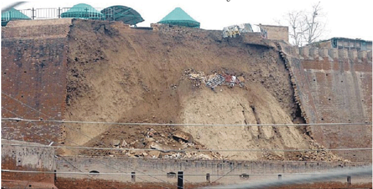
(c) Peshawar City, Fort: Collapse of masonry retaining wall and backfill sliding of Fort "Qilla Bala Hisar".
