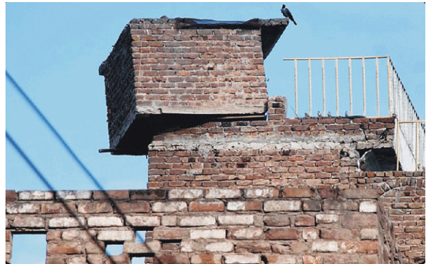
(b) Peshawar City, Ganj: Sliding of overhead tank on the building roof.
