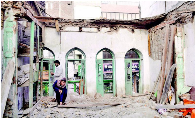
(a) Peshawar City, Qisa Khwani Bazar: Complete collapse of building roof.
