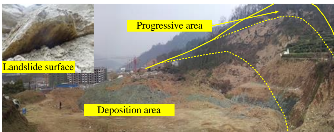
Fig. 3. Landslide YYG03 caused by slope cut in the residential quarter of Yuyanguan.
