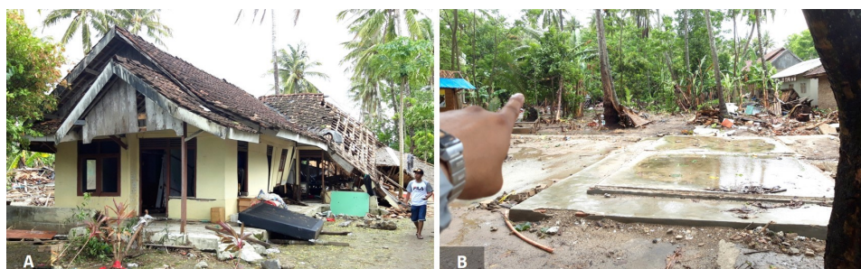
Fig. 13. Examples of damages at wooden houses: (a) Major damages and (b) complete damage/washed away.
