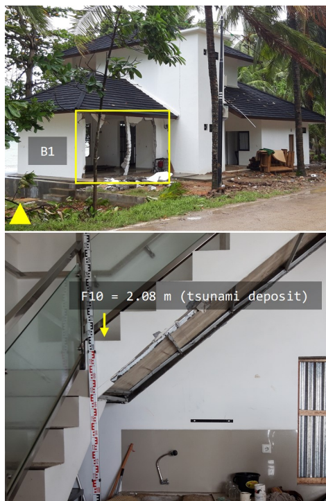
Fig. 4. A villa's wall destroyed by tsunami in Bulukan Pondok beach (left) and a 2.08 m of flow depth recorded on the stair inside the villa (right). One story house had a major damage, meanwhile the two-storeys house was moderate.
