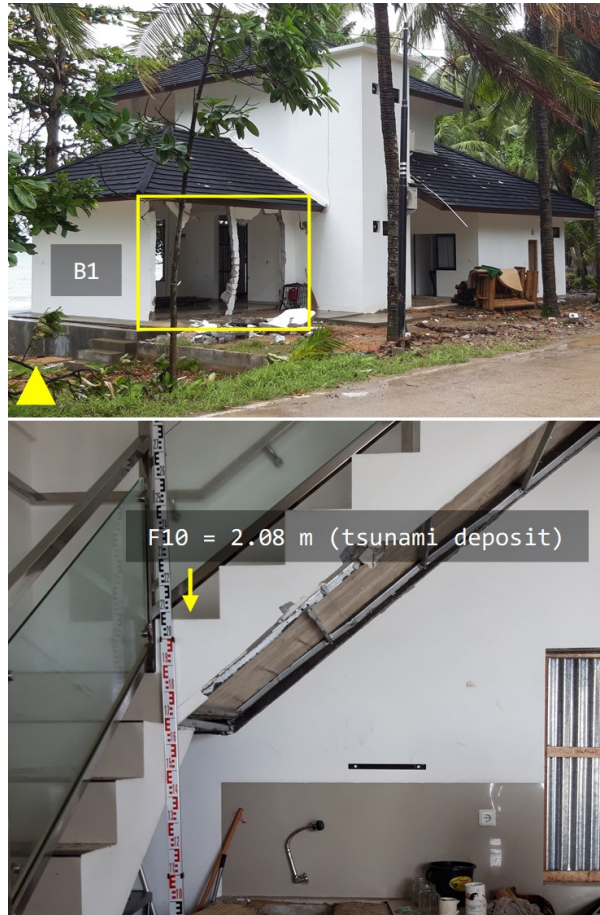
Fig. 4. A villa's wall destroyed by tsunami in Bulukan Pondok beach (the upper figure) and a 2.08 m of flow depth recorded on the stair inside the villa (the lower figure). One story house had a major damage, meanwhile the two-storeys house was moderate.
