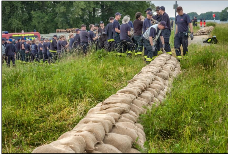
Figure 2: Firemen during the Elbe flood in 2013. Setting up a sandbag dam to raise a dyke.
