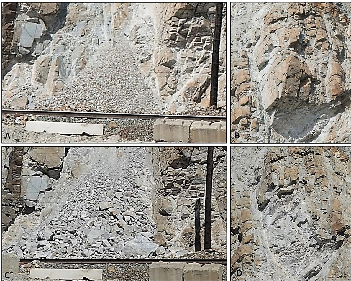
Figure 8: Before and after photos of the 24 m 3 wedge sliding event from White Canyon East, Site B. The top row of photos shows the pre-fall debris present in the track-side ditch (A), as well as the pre-fall source zone (B). The bottom row shows the post-fall accumulation in the track-side ditch (C), as well as the post-fall source zone (D). From these images we can see the heavily jointed state of the rockfall mass pre-fall and the rockfall back-scarp, post-fall. A notable increase in the quantity and size of debris fragments in the track-side ditch is visible post-fall.
