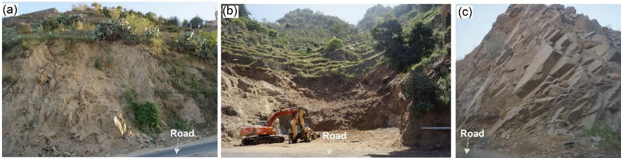
Figure 5. Landslides proximal to, possibly triggered by, road construction and intensified by rainfall (a) Debris flow caused by failure on steep slopes intersected by roads. (b) Debris flow caused by failure of terraces constructed on steep slopes. (c) Landslide caused by failure on fracture planes dipping towards the road.
