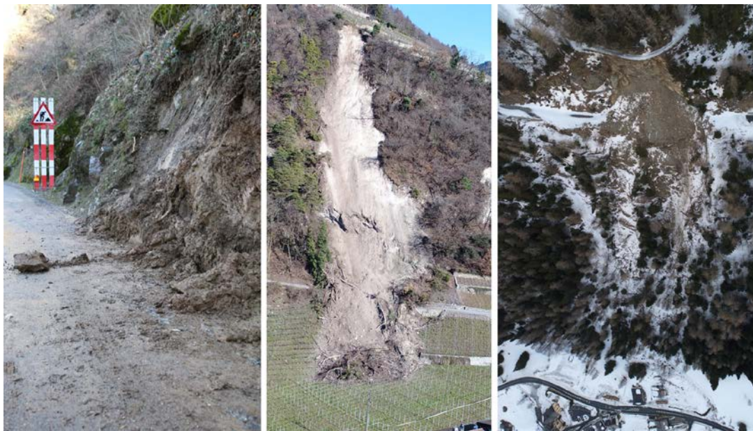
346 347 Figure 4: Examples of events affecting roads. Left: small event already removed but still unstable on the 348 uniquely accessible road to the small village of Morcles (Canton of Vaud). Middle: middle event on a minor 349 road in Ollon (Canton of Vaud). Right: large event with a volume estimated at 3500 m 3 that cut a 50 m length on
