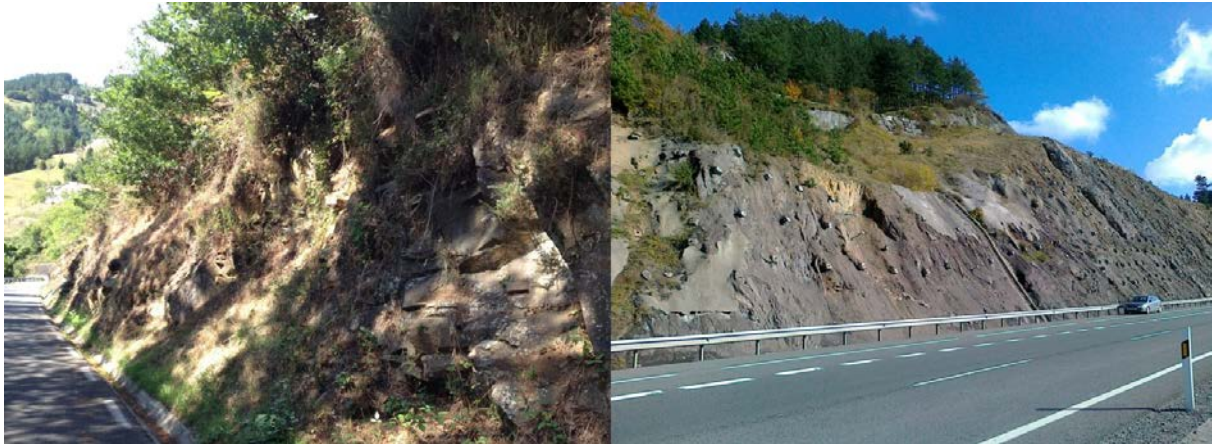
5 Figure 7: (left) PoR L1C of the road GI-3324 (from km 0.700 to 1.450), without protection measures; (right) PoR P4C of the road N-1 (km 407.395 to 407.680) with protection measures.
