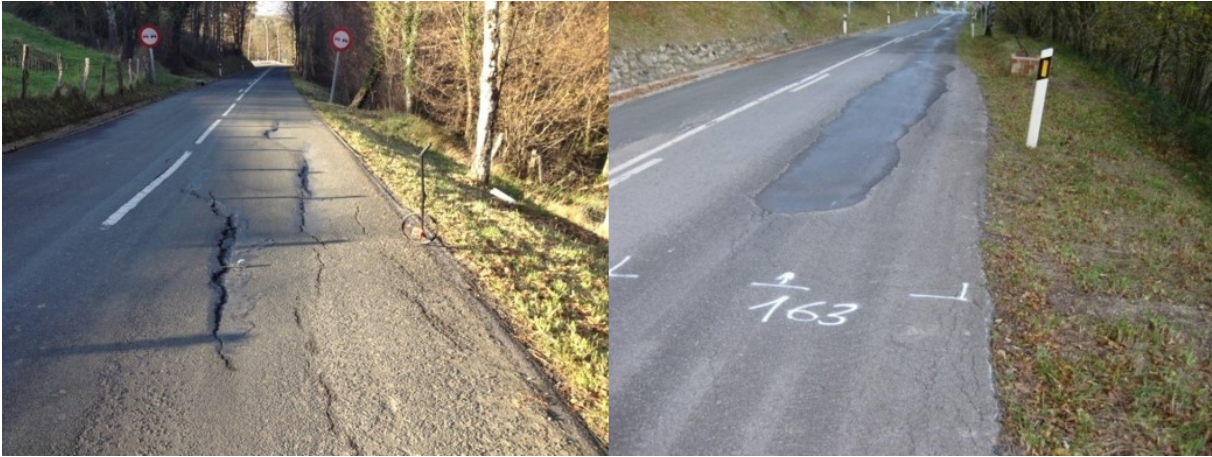
25 Figure 9: Road sections situated within slow moving landslides, with damage: (left) PoR C3C of the road GI-2133 (from km 8.280) with observed deformations and cracks on the road pavement; (right) PoR C9G of the road GI2637 (from km 17.891 to 18.220) showing minor cracks already sealed.
