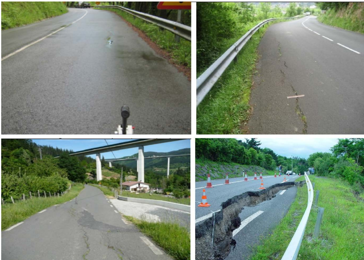
20 Figure 5: The four damage levels identified at the roads of Gipuzkoa: (top-left) No/Slight damage, (top-right) Moderate damage, (down-left) Severe damage, and (down-right) Partial/total destruction.
