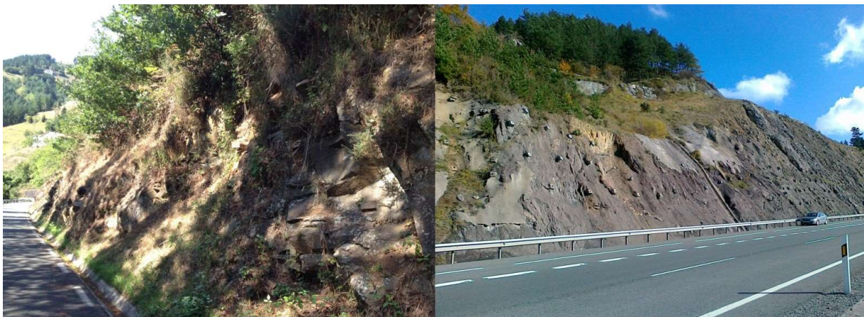
Figure 7: (left) PoR L1C of the road GI-3324 (from km 0.700 to 1.450), without protection measures; (right) PoR P4C of the road N-1 (km 407.395 to 407.680) with protection measures.
