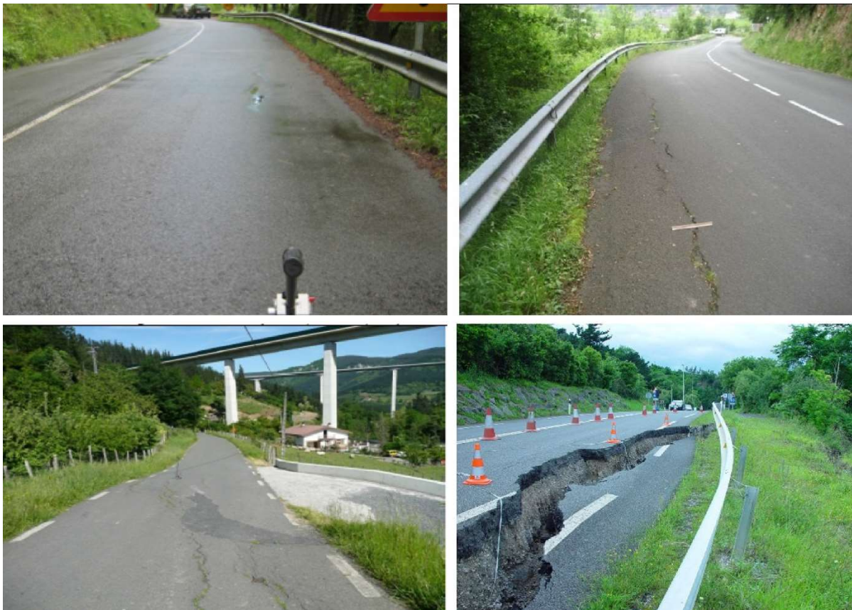
20 Figure 5: The four damage levels identified at the roads of Gipuzkoa: (top-left) No/Slight damage, (top-right) Moderate damage, (down-left) Severe damage, and (down-right) Partial/total destruction.
