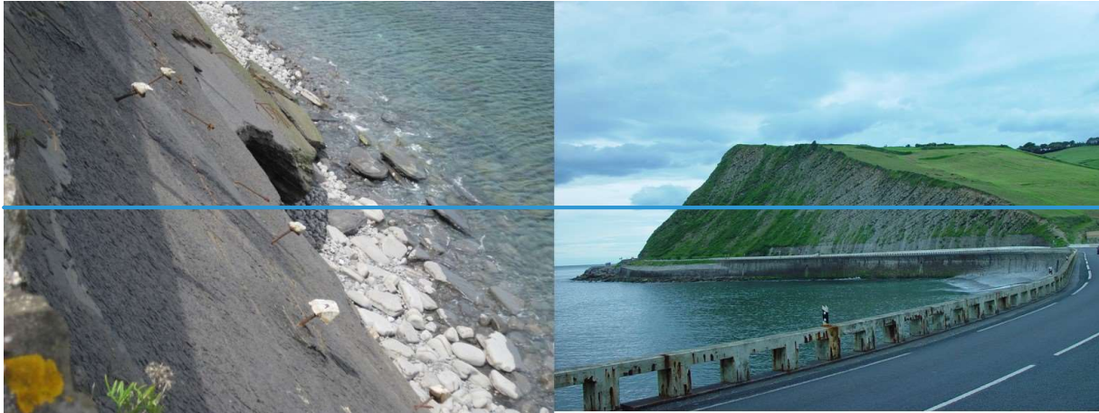
Figure : (left) PoR B9A of the road GI 638 (from km 1.400), of high risk, with a view of the coastal wall from the road, with oxidised and bent bolt. The sea wave action has left the rock exposed and the bolt unsupported; (right) PoR P7L of the road N 634 (from km 24.650 to 24.750), which was stabilized in May 2014.
