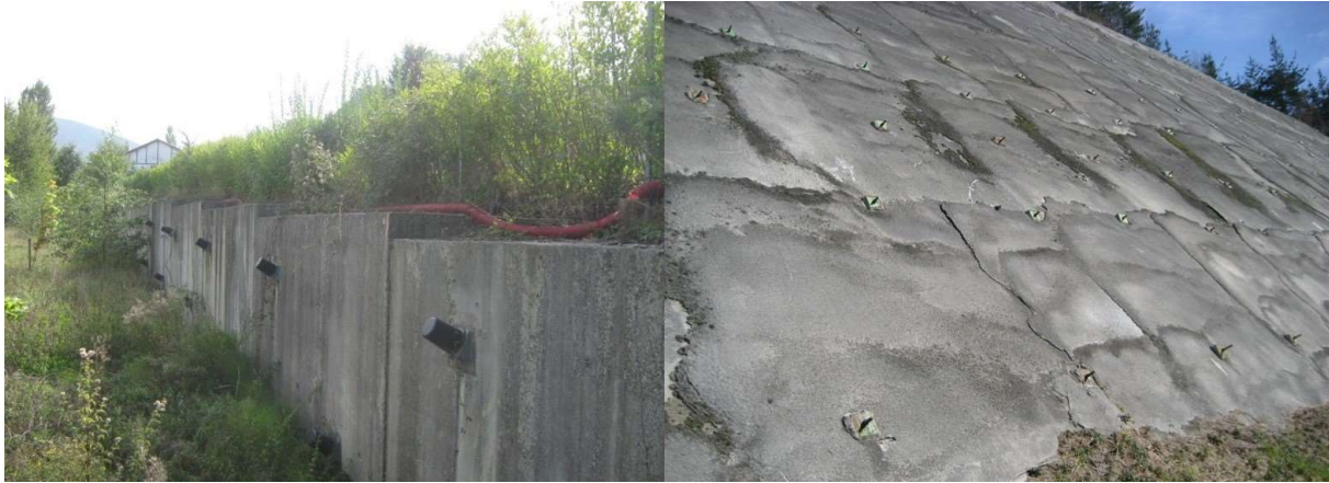
Figure 8: (left) PoR P2A of the road AP-8-1-1 (from km 77.140 to 77.210) where the crest of the slope and the retaining wall with anchors is seen; (right) C8A of the road G-2634 (32.980 to 33.150) with gunite, rock bolts, and anchors.
