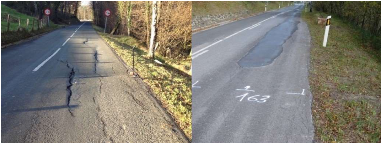
10 Figure 9: Road sections situated within slow moving landslides, with damage: (left) PoR C3C of the road GI-2133 (from km 8.280) with observed deformations and cracks on the road pavement; (right) PoR C9G of the road GI2637 (from km 17.891 to 18.220) showing minor cracks already sealed.
