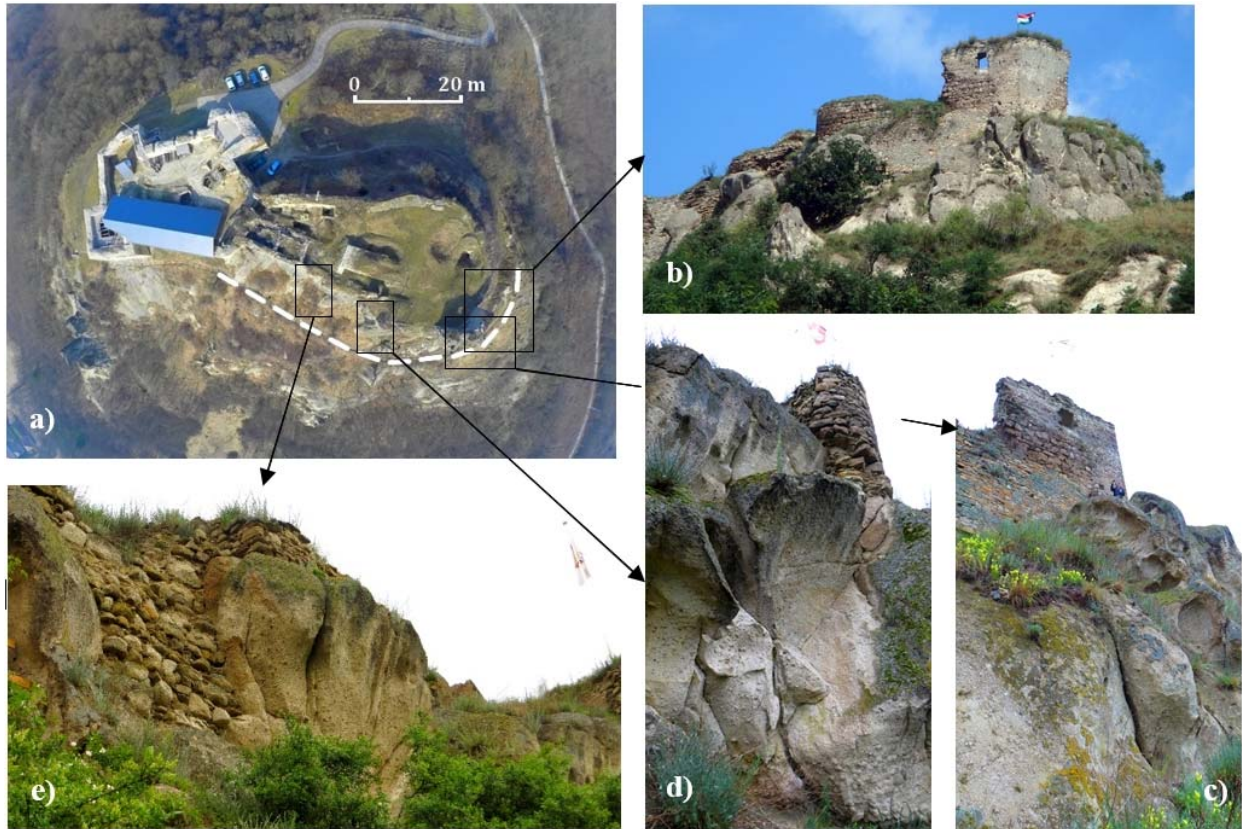
Fig.2. Studied southern cliff faces (clockwise): a) image of the castle obtained by RPAS with marked details; b) distant view of the eastern part of the cliff section; c) weathered rounded cliff with larger taffoni; d) vertical to sub-vertical cliff face with steep joints and traces of rock fall; e) steep cliffs dissected by joints.
