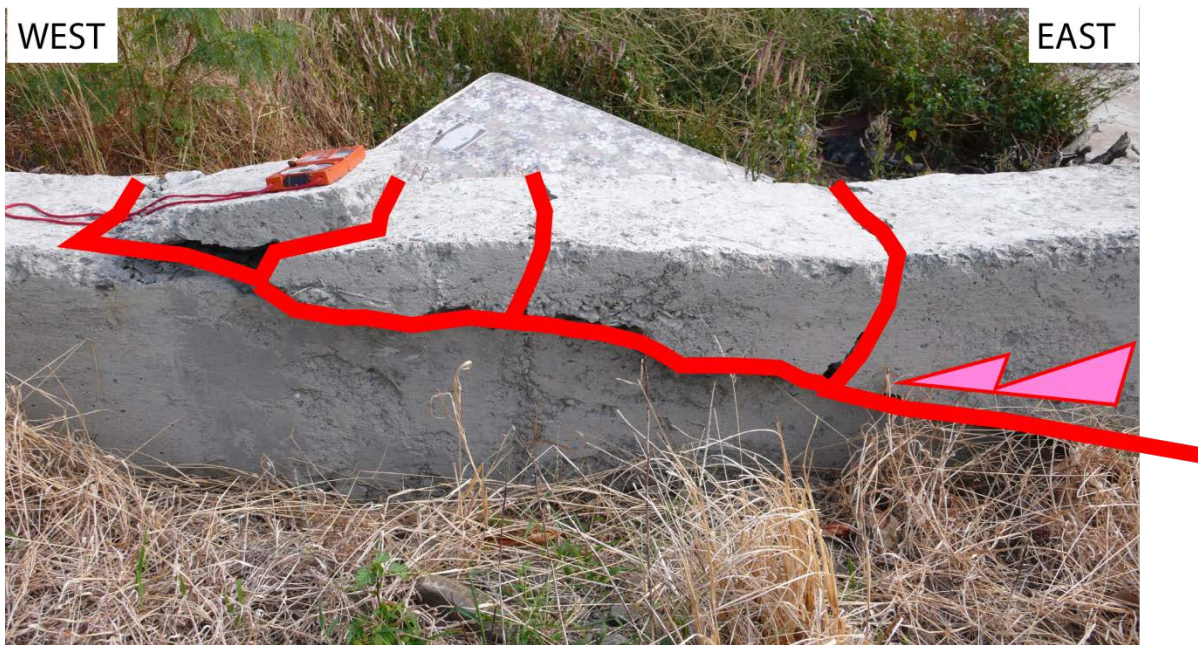
5 Figure 5: Field work photograph of compressive features affecting recent concrete dykes after the Hengchun earthquake (Dec. 26 th 2006, M_L=7.0 ), see location on Fig. 1 near the Fang-Shan village ( 22.26^\circ\text{N} , 120.66^\circ\text{E} ). The red compass gives the scale of the outcropping deformation (20cm). Thrust associated with three back-thrusts highlighting a small pop-up (below the compass). The red arrow reveals the thrusting component that affects the new concrete dykes
