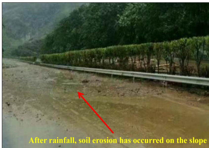
Figure 2. Soil erosion produced by rainwash on slope
