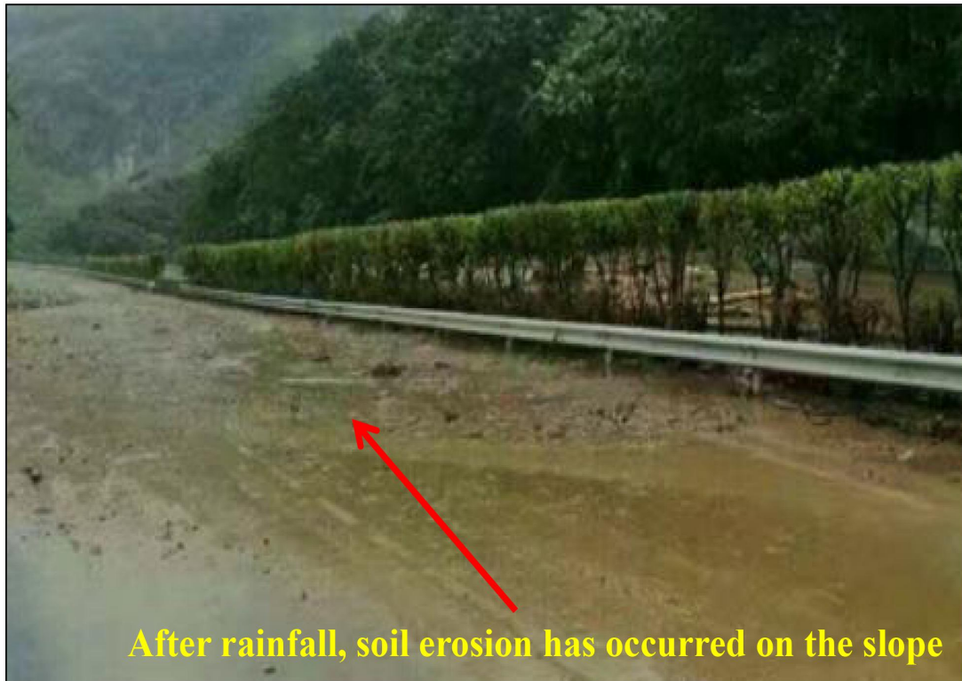
Figure 1. Soil erosion produced by rainwash on slope
