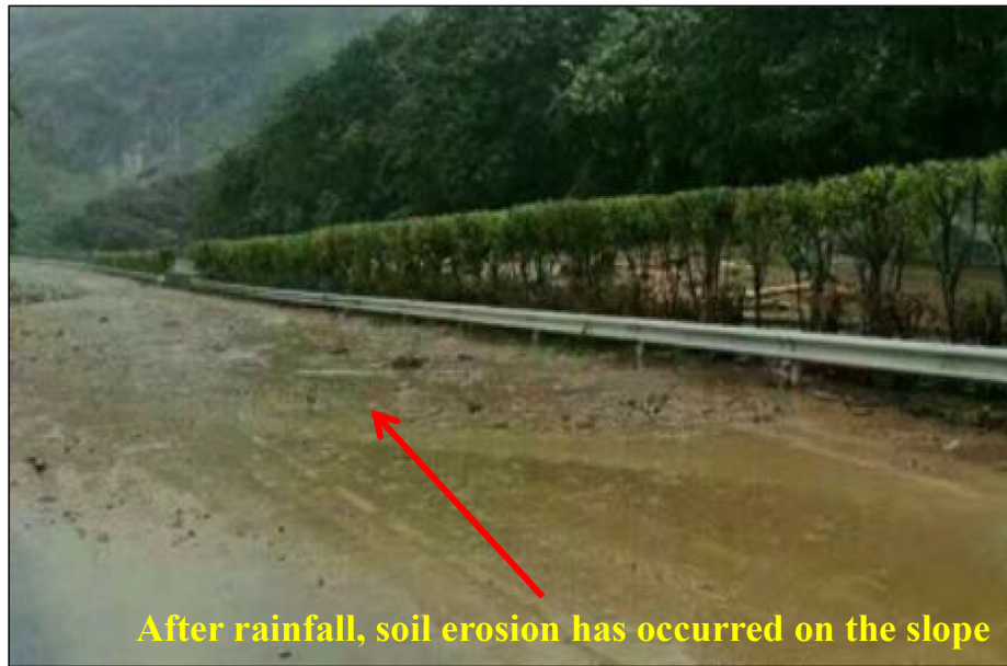
Fig. 2. Soil erosion produced by rainwash on slope
