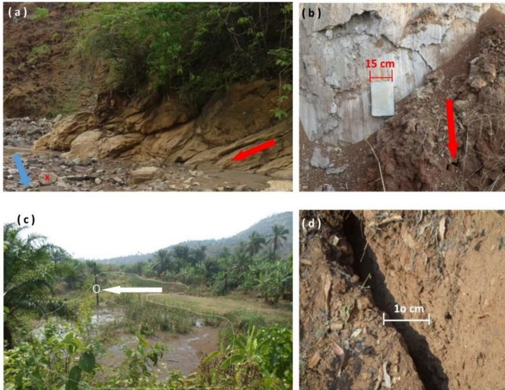
Figure 3. Field observations highlighting the critical stability state of BTL. (a) View of the rock structures at the foot of the landslide (note the boulder marked by a red cross in the lower left part has a diameter of about 60 cm), generally dipping towards the north (left side), parallel to the sliding direction (red arrow). The blue arrow indicates the river flow direction. (b) View of a crack on the sliding interface in clay. The red arrow shows the direction of sliding of the right part along the clay layer. (c) Pond on the landslide with an oil palm tree designated by the white arrow. This shows that these ponds are recent (oil palm trees do not grow in water; its particular foliage compared to others shows that its growth was stopped recently). (d) A crack found on the landslide surface.
