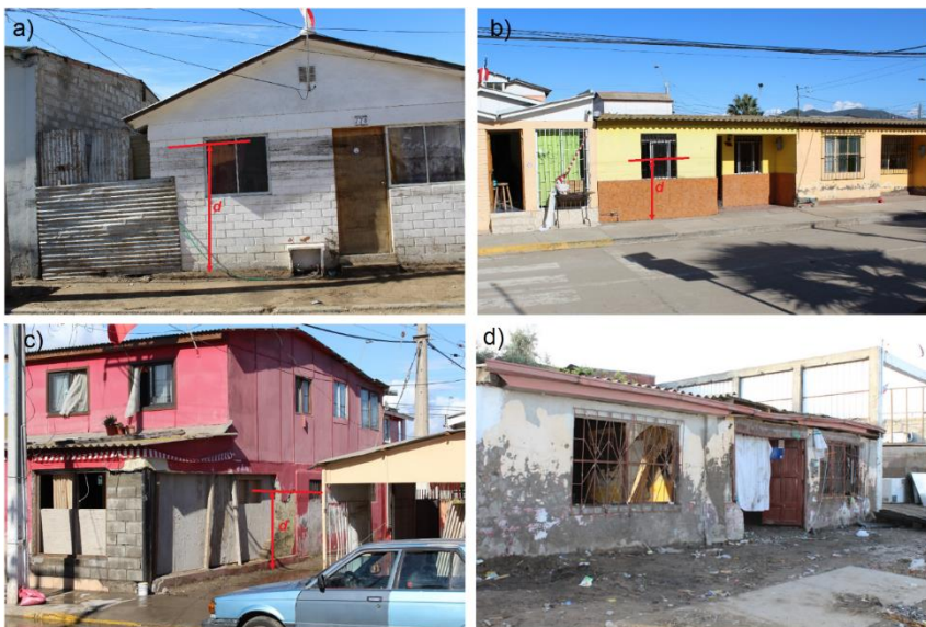
Figure 2: Photographs of structures undamaged and damaged by the 2015 tsunami in the Coquimbo area. The red letter d indicates the observed tsunami flow depth.
