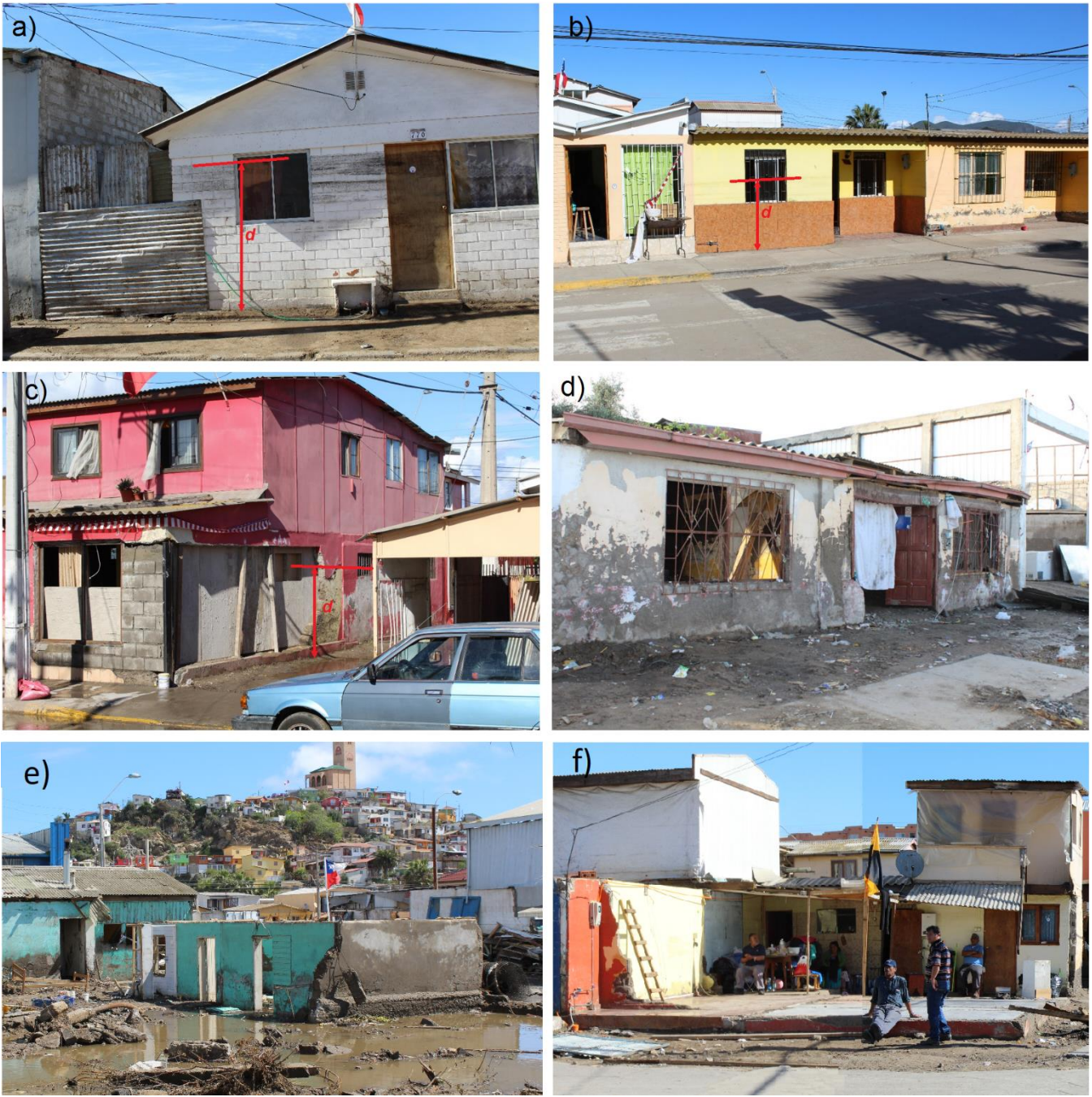
Figure 2: Photographs of surveyed masonry houses after by the September 16 th 2015 tsunami in the Coquimbo area. The red letter d indicates the observed tsunami inundation flow depth . All photos were taken on September 22 nd of 2015. a) and b) Houses with no damage. c) 2-story house with moderate damage. d) 1-story house with major damage. e) 1-story house with complete damage. f) Washed away structure.
