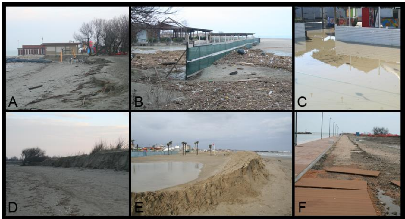
Figure 3: Impacts of the event in February 2015 on the Lido degli Estensi-Spina case study area. Impacts of erosion and flooding on concessions at Lido di Spina south (A, B) and Lido degli Estensi (C); sandy scarp due to the erosion of the dune in the south of Lido di Spina (D); eroded Winter Dune in Porto Garibaldi (E); damages to the Porto Canale front at the Lido degli Estensi (F).
