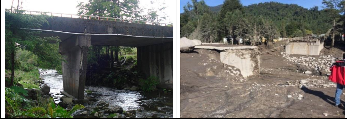
Figure 2: (a) Original Río Blanco Bridge (Chile) (MOP, 2015). (b) Río Blanco Bridge (Chile) after lahar flow of the Calbuco volcano eruption in 2015 (MOP, 2015).
