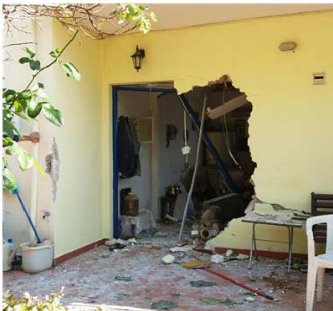
Figure 3. Impact of rock on house in Ponti, Lefkada, Greece.
