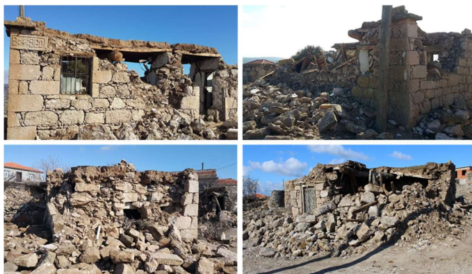
Figure 14 Examples of heavy earth wall collapse
