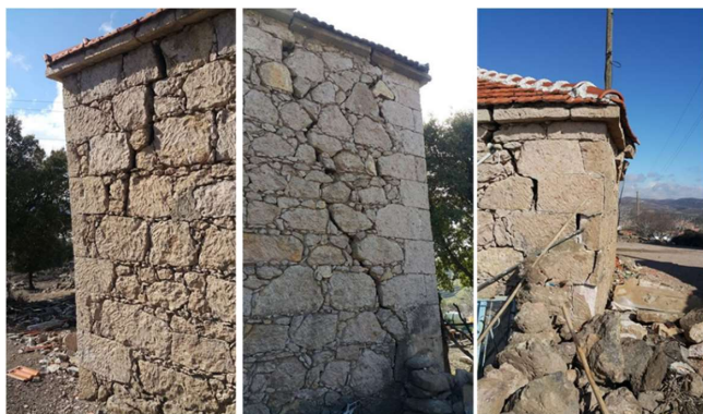
Figure 16 Examples of diagonal shear cracking
