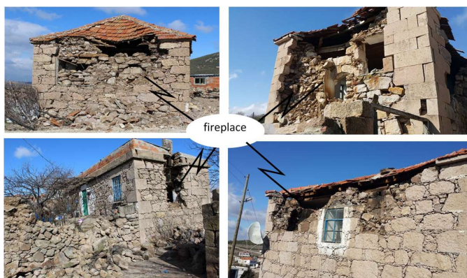
Figure 13 Examples of out of plane collapse due to wall cavity
