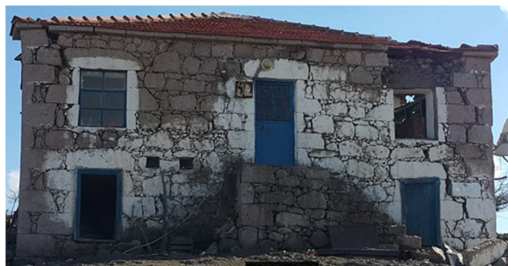
Figure 10 An example of damaged dwelling due to inadequate interlocking
