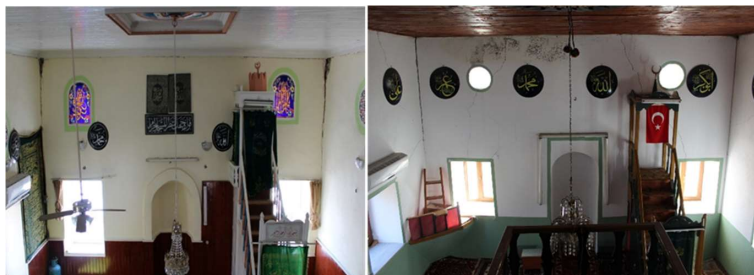
Figure 12 Observed damages at intersection of perpendicular walls
