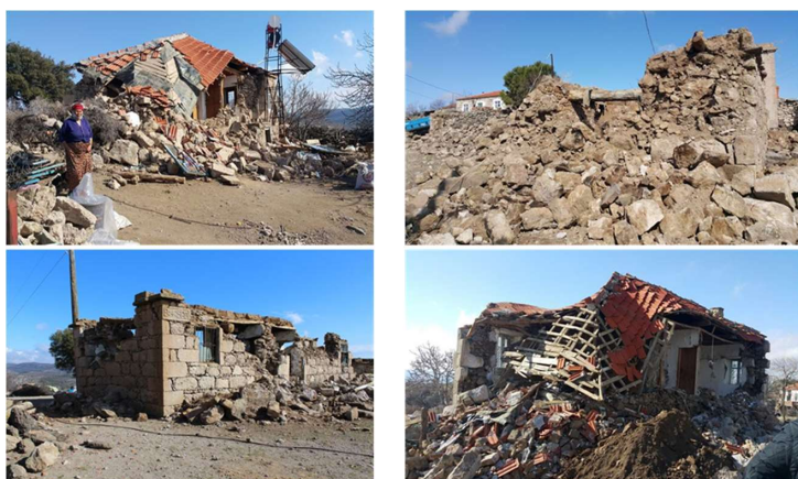
10 Figure 9 Totally collapsed examples from Ayvacık, Çanakkale 2017 earthquakes swarm
