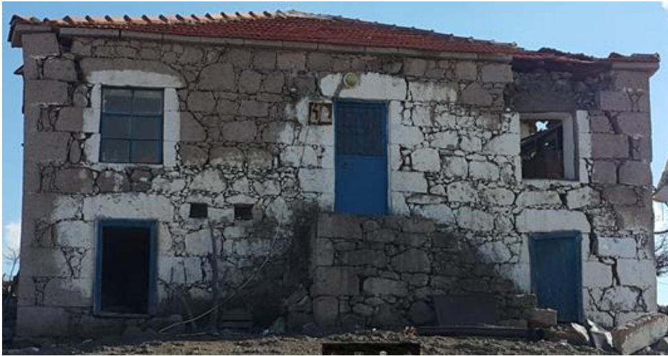
Figure 17: An example of a damaged dwelling due to inadequate interlocking
