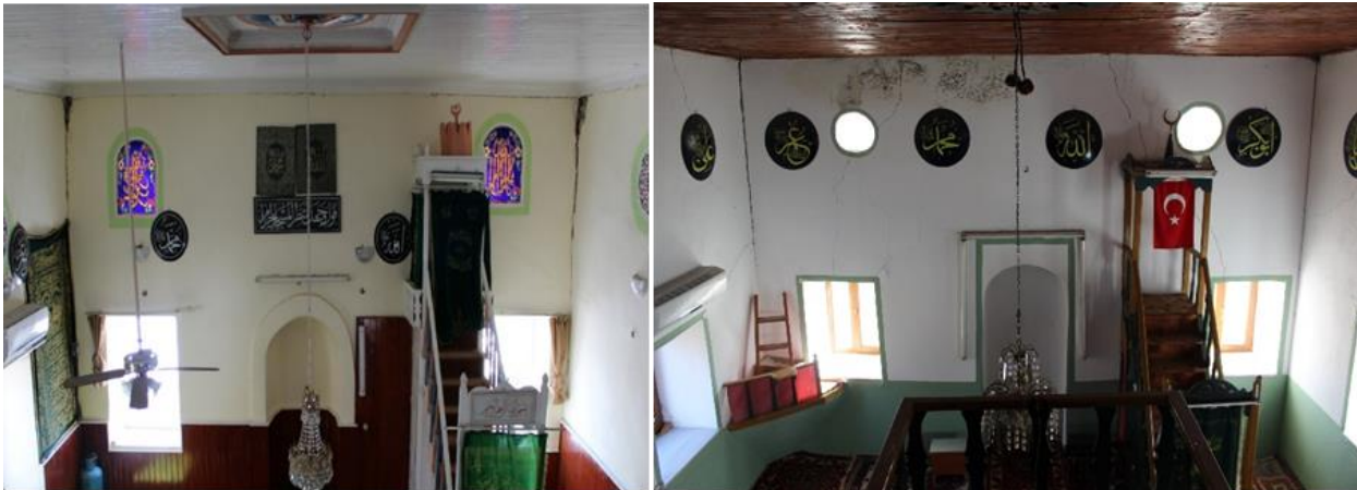
Figure 19: Observed damages at intersection of perpendicular walls
