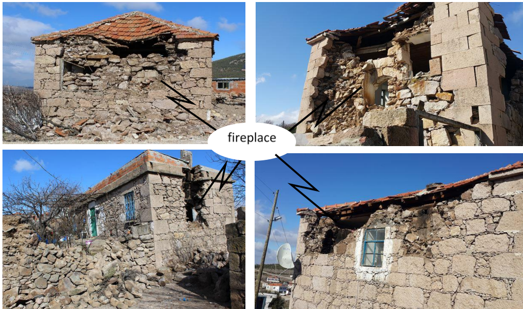
Figure 20: Examples of out of plane collapse due to wall cavity
