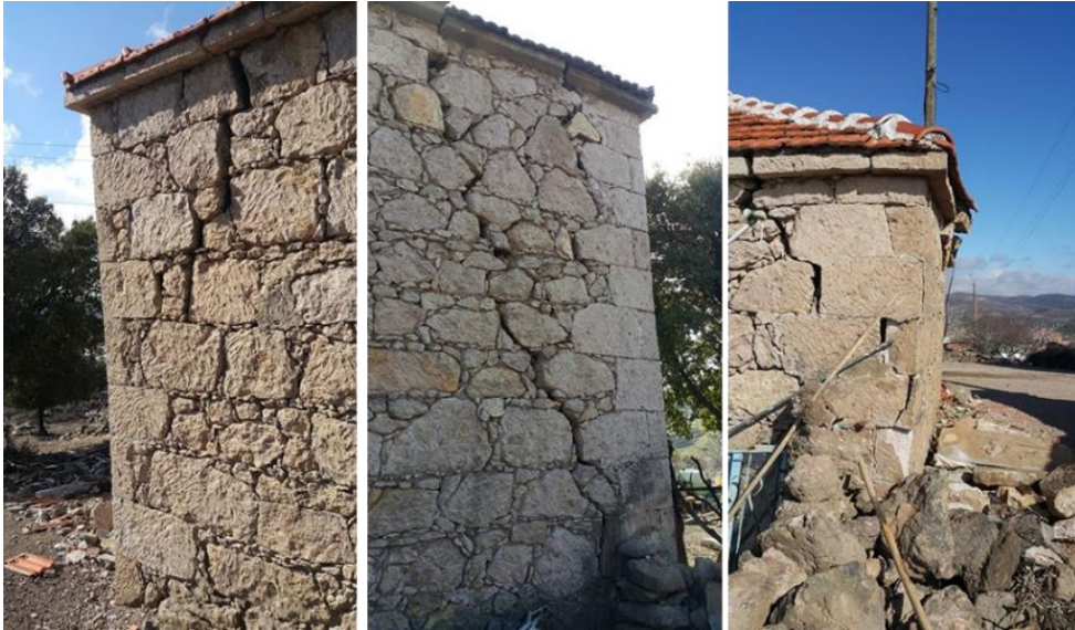
Figure 23: Examples of diagonal shear cracking
