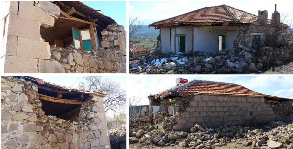
10 Figure 24: Out of plane failures due to improper wall thickness and/or height-length ratio
