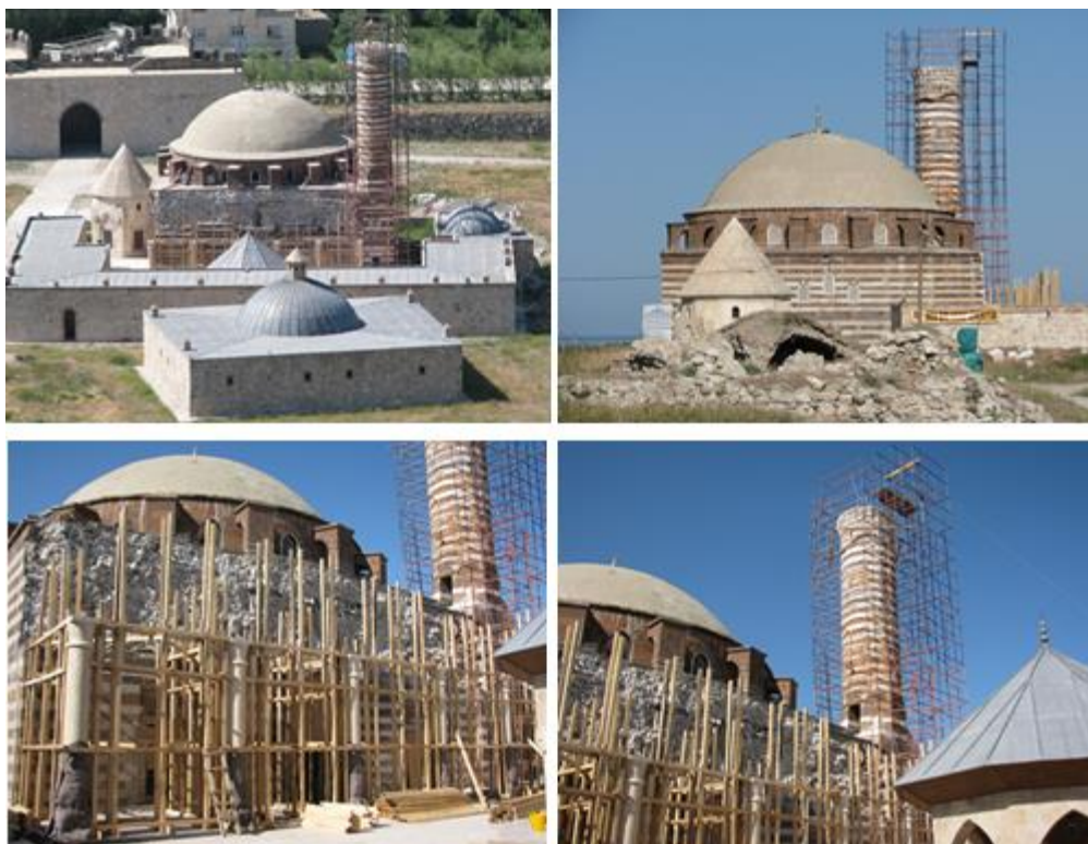
5 Figure 3: Damaged views and dangerous cases of Hüsrev Pasha Mosque.
