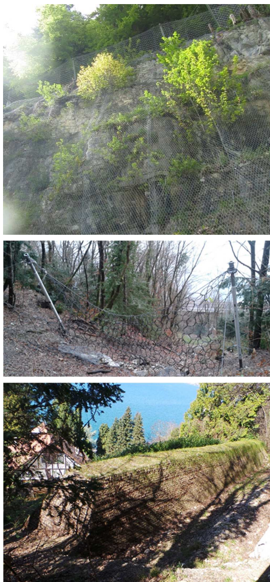
5 Fig. 2. Protection measures installed on the slopes above the city of Montreux (Switzerland). Above: barrier fences and cable nets on the cliff overhanging the Cantonal Road near the town of Vallorbe. Centre: barrier fence (Source: Grisanti and Prina Howald, 2015). Below: earth dam (Source: Privat and Prina Howald, 2014).
