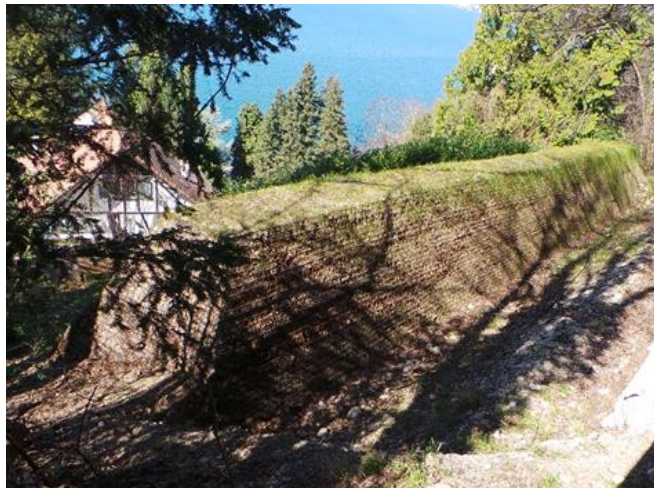
5 Fig. 2. Protection measures installed on the slopes above the city of Montreux (Switzerland). Above: barrier fences and cable nets on the cliff overhanging the Cantonal Road near the town of Vallorbe. Centre: barrier fence (Source: Grisanti and Prina Howald, 2015). Below: earth dam (Source: Privat and Prina Howald, 2014).
