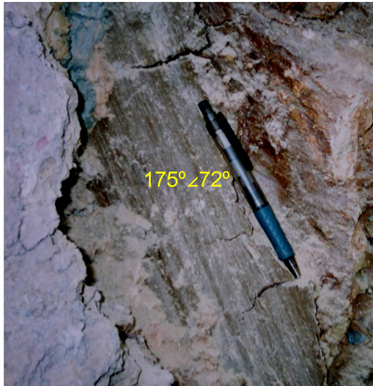
Figure 15. The sliding scrape of the scarp be revealed by foundation excavation.
