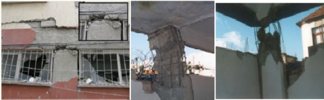
Figure 10. Examples of damage caused by the formation of short columns [8].
