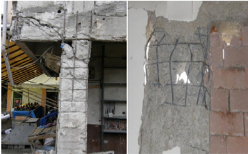
Figure 17. Damage caused by excess stirrup intervals in the confinement zones of columns [20].
