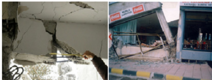
Figure 15. Pulling away of longitudinal reinforcements.
