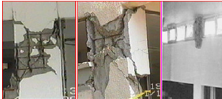
Figure 9. Several short column failures observed after earthquakes [5].
