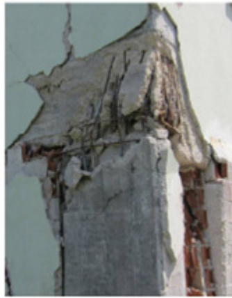
Figure 14. A reinforced concrete structure that was heavily damaged at the integration region during the May 19, 2011, Simav Earthquake [10].
