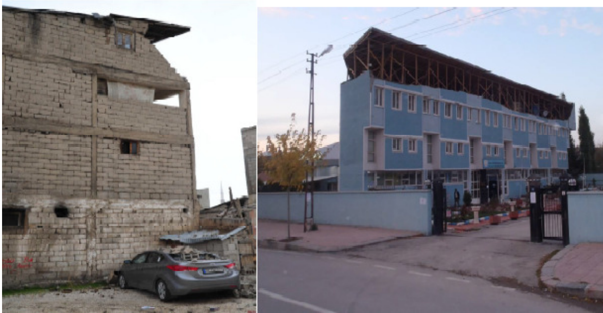
Figure 24. Gable wall damage ( www.dramaistanbul.com.tr ).
