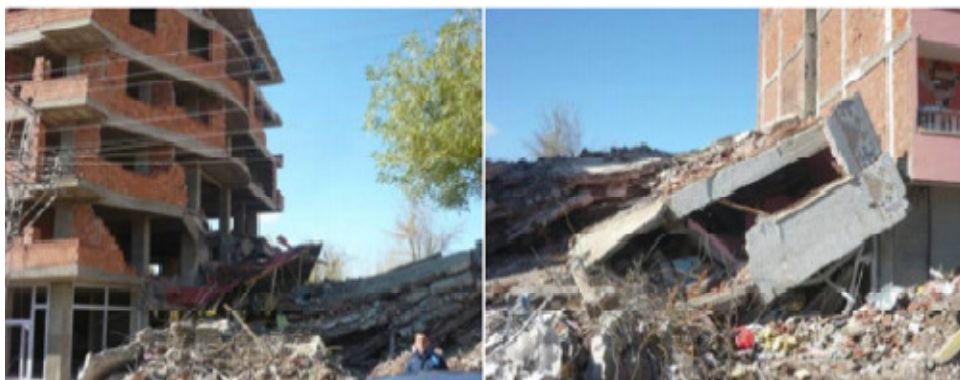
Figure 26. Reinforced concrete multi-story building that collapsed by colliding with adjacent buildings due to a daubling effect [15].
