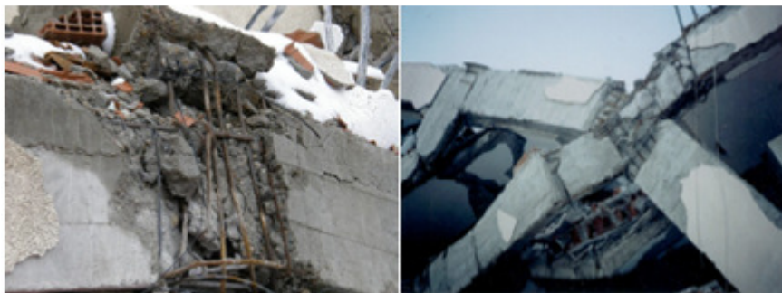
Figure 18. Damage to column-beam joint region [20].
