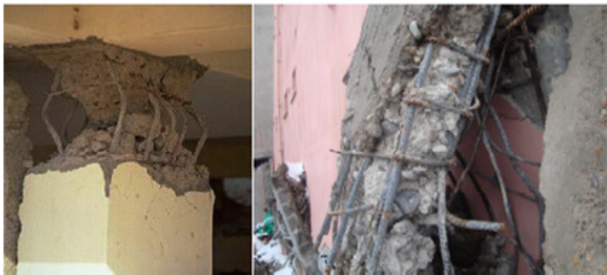
Figure 16. Damage caused by reinforcement detailing mistakes (Source: Erdal Camcı).
