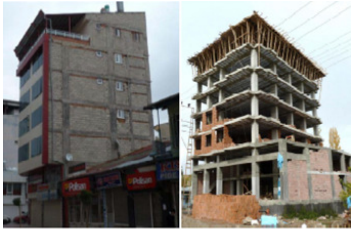
Figure 21. Buildings that do not have adequate shearwalls.
