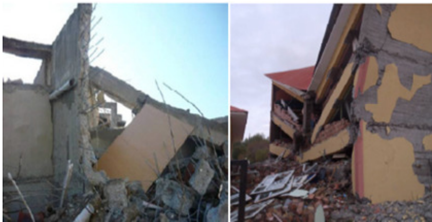
Figure 25. A building that collapsed due to contributions of lateral translation and torsion [3].
