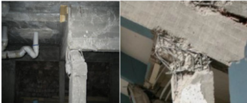
Figure 19. Examples of strong beam-weak column damage.
