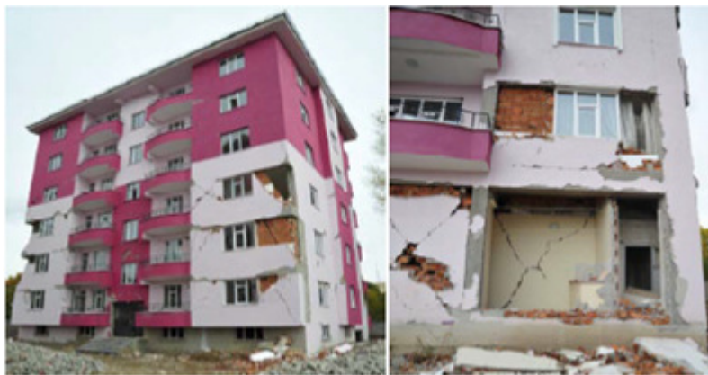
Figure 23. Damage observed in non-bearing brick-infilled walls.
