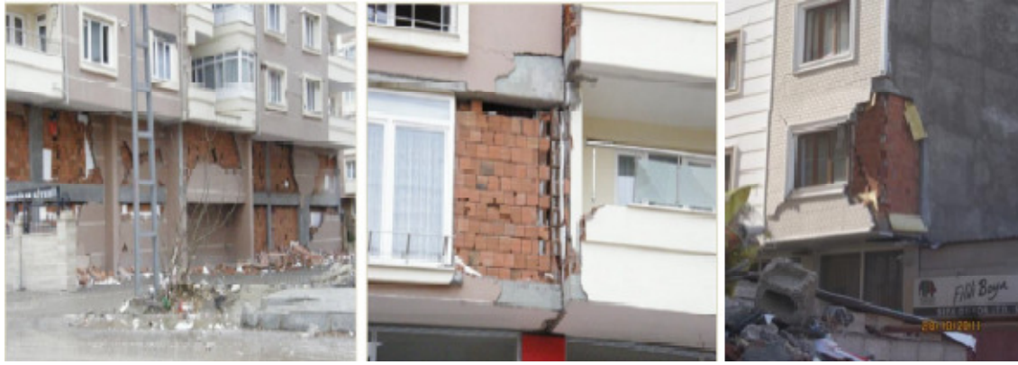
Figure 27. Damage in the outer walls of a reinforced concrete building in Van city due to separations in the walls [16].
