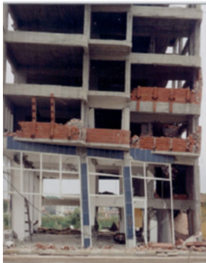
Figure 13. Heavy damage in the weak story of a five-floor building in Adapazari (August 17, 1999, Kocaeli Earthquake, M = 7.4 ) [5].
