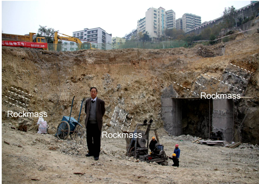
Figure 25. Rockmass showing their anomalous attitudes each other in the western wall of the foundation pit, and this kind of geologic structure is only generated by landslides.
