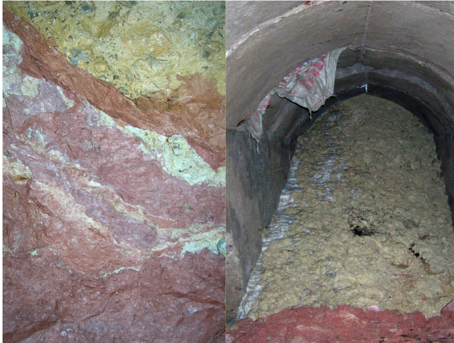
Figure 17. The sliding zone and slip mass in tunnel near by the eastern lateral edge.
