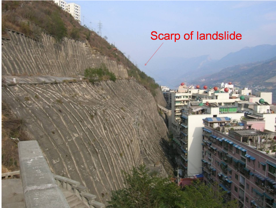
Figure 14. The scarp of the Sanmashan landslide (March 2006).
