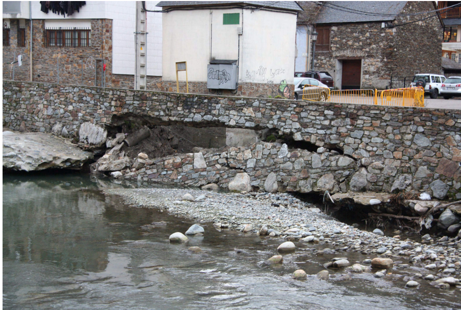
Figure 12. Collapse of a channelization dyke at Les due to vertical incision (photo Glòria Furdada, 15 January 2014).
